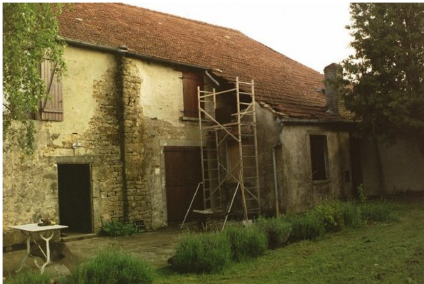
afb. 07.2 - 4 Bij de lekkende goot was de pleister al weg. --> Under a leaking gutter the plaster was already degraded.
