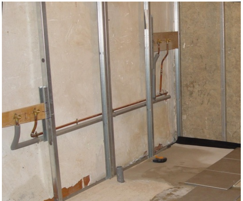
afb. 07.1.1 - 20 Badkamerleidingen (links badkuip, rechts douche) achter de ossature -> bathroom copper piping behind the uprights (left: bath, right: shower)
