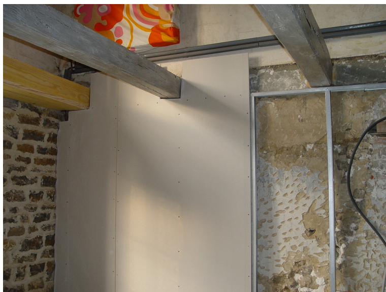
afb. 07.1.1 - 24 Gipsplaten rond de balken uitgesneden, spleten van 5 à 8mm -> plasterboard cut out around the beams with gaps of 5 - 8mm (isn't that 3/16 to 5/16"?)
